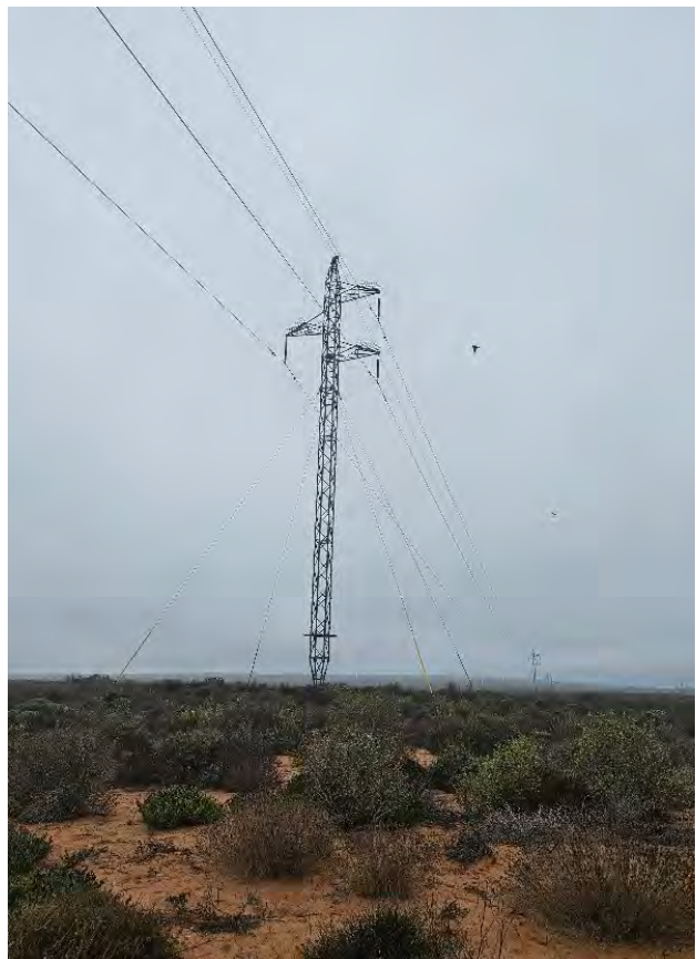
Field site near the Sere Windfarm and the monitored powerline (Photo: Yusra Samsodien).
