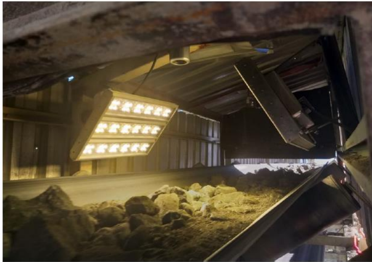
Figure 4.3: Camera and floodlight installation at Kao Diamond Mine, above the primary feed conveyor.
