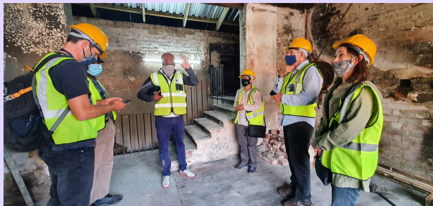
Senior Science Faculty staff inspecting the damage to Science Faculty Buildings soon after the fire
