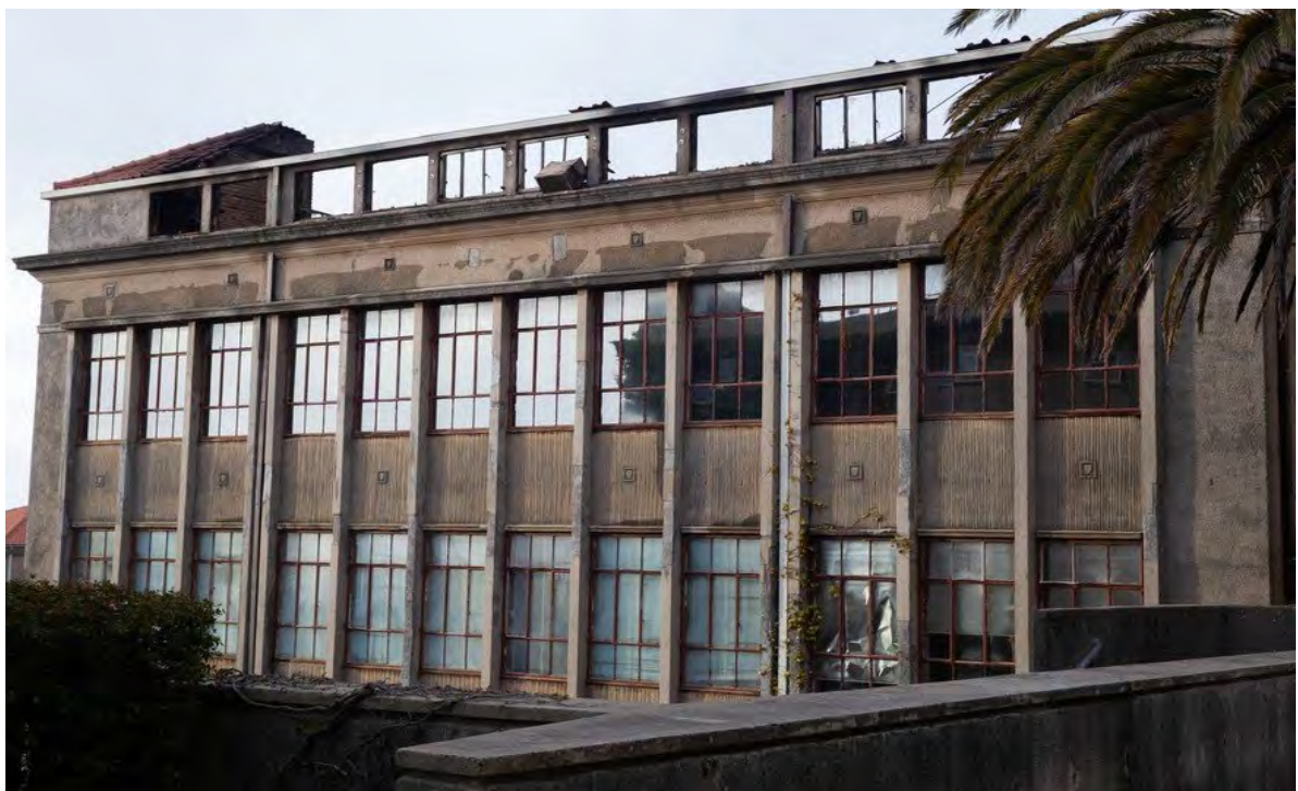
The former home of the Fitz atop the HW Pearson Building, which currently houses the Plan Conservation Unit, was gutted by the fire on 18 April 2021 (Photo: News24).
